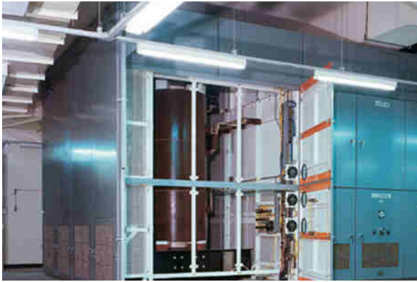
Transformer cubicle for substation in building
